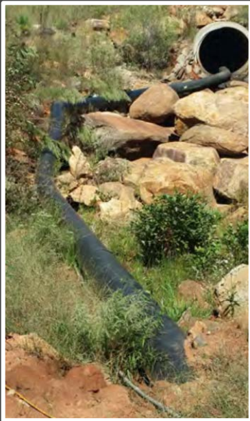
16" penstock from upper lake
